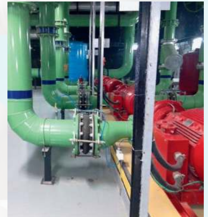
Easyflex Single Arch Rubber Bellows with CHW Pumps for HVAC System.
