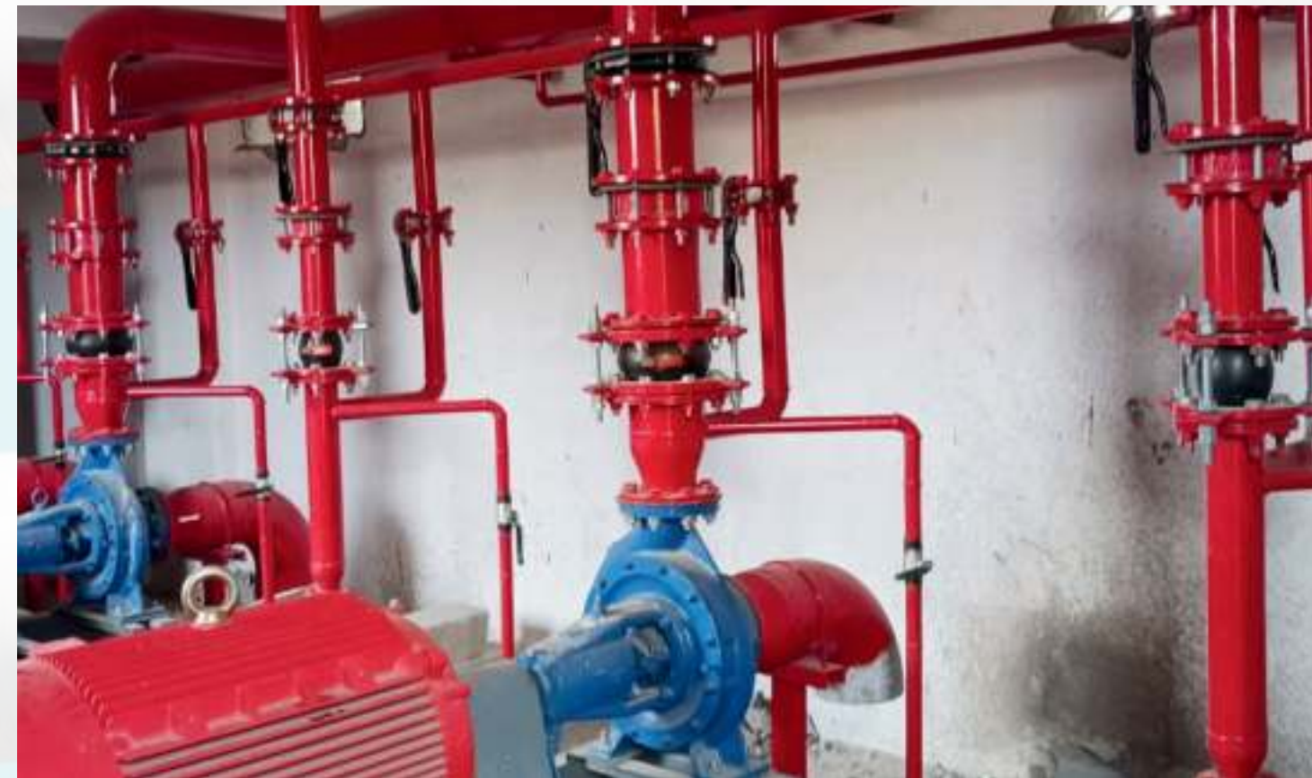
Easyflex Rubber Expansion Joints PN20 with Swivel Flanges and Control Unit Assembly for Fire Fighting system.
