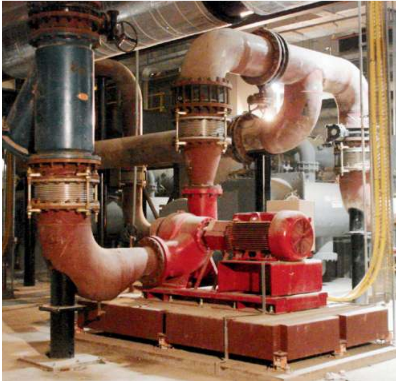
Easyflex Metallic Expansion joints fitted with CHW Pump ; installed on Easyflex Inertia Base with Seismic Mounts.
