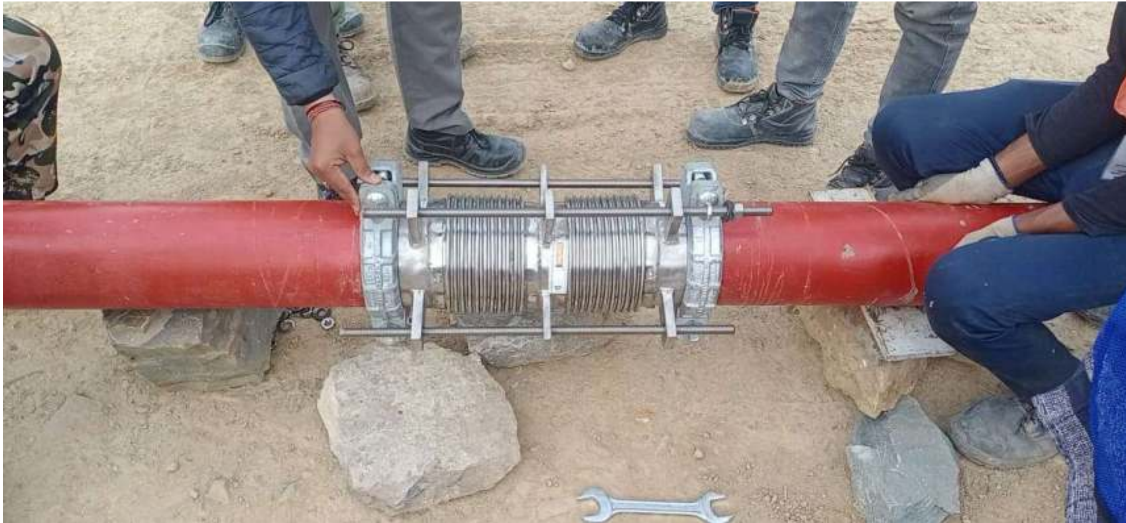
Easyflex Universal Expansion Joint with Grooved Pipe Ends installed at Fire piping for a Tunnel Project.
