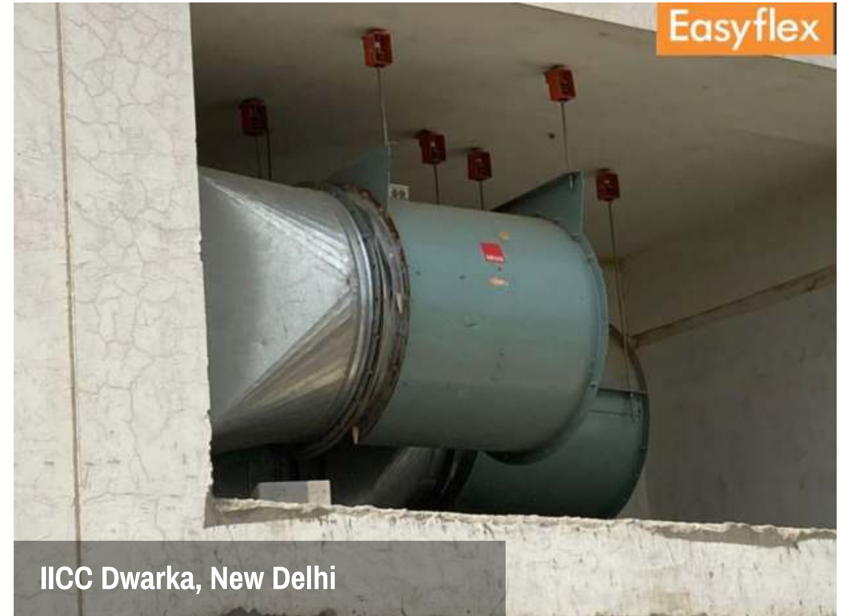
Axial Fans installed with Spring Hangers and Flexible Duct Connectors
