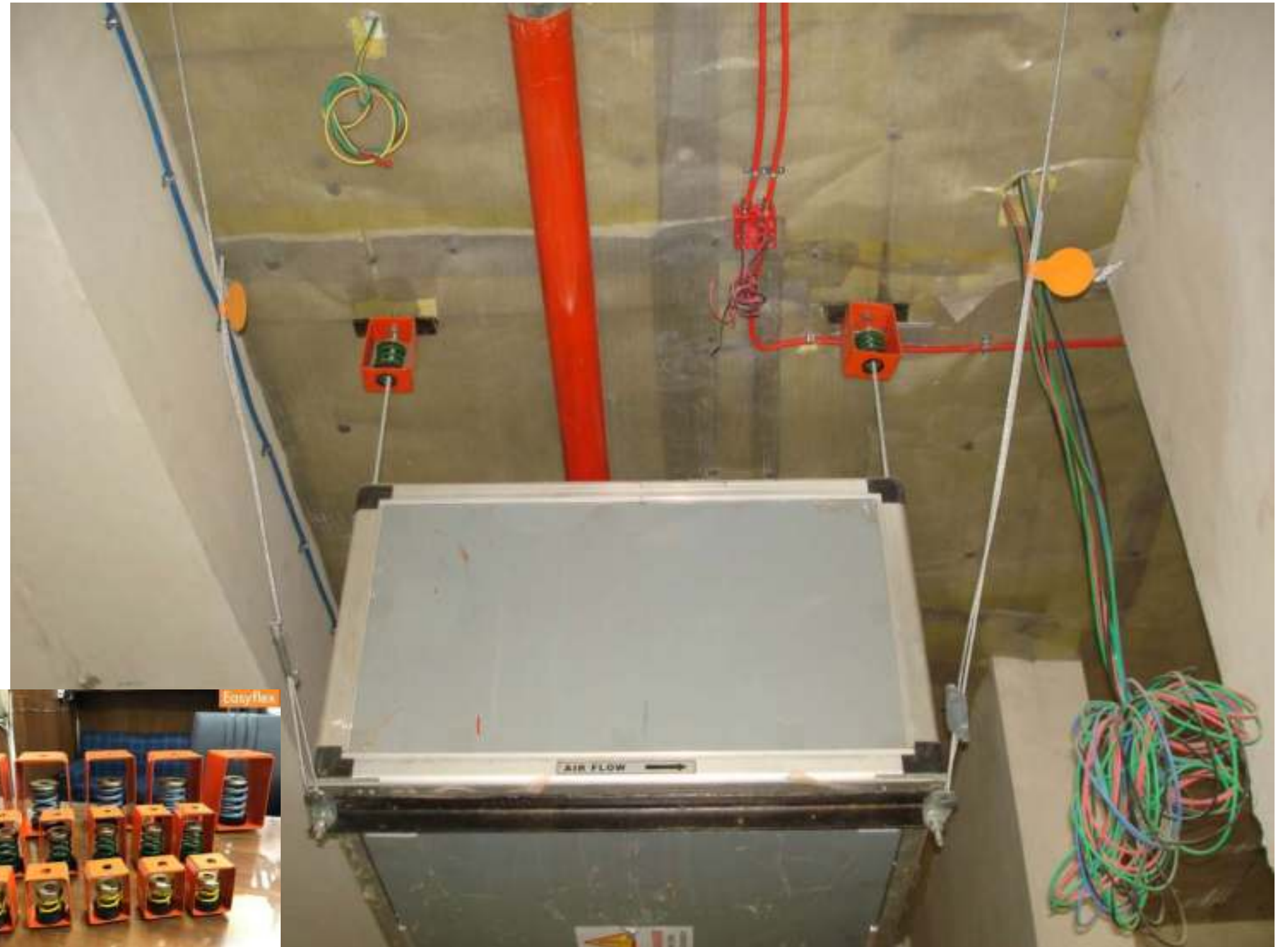
Fan Coil Unit installed with Spring Hangers
