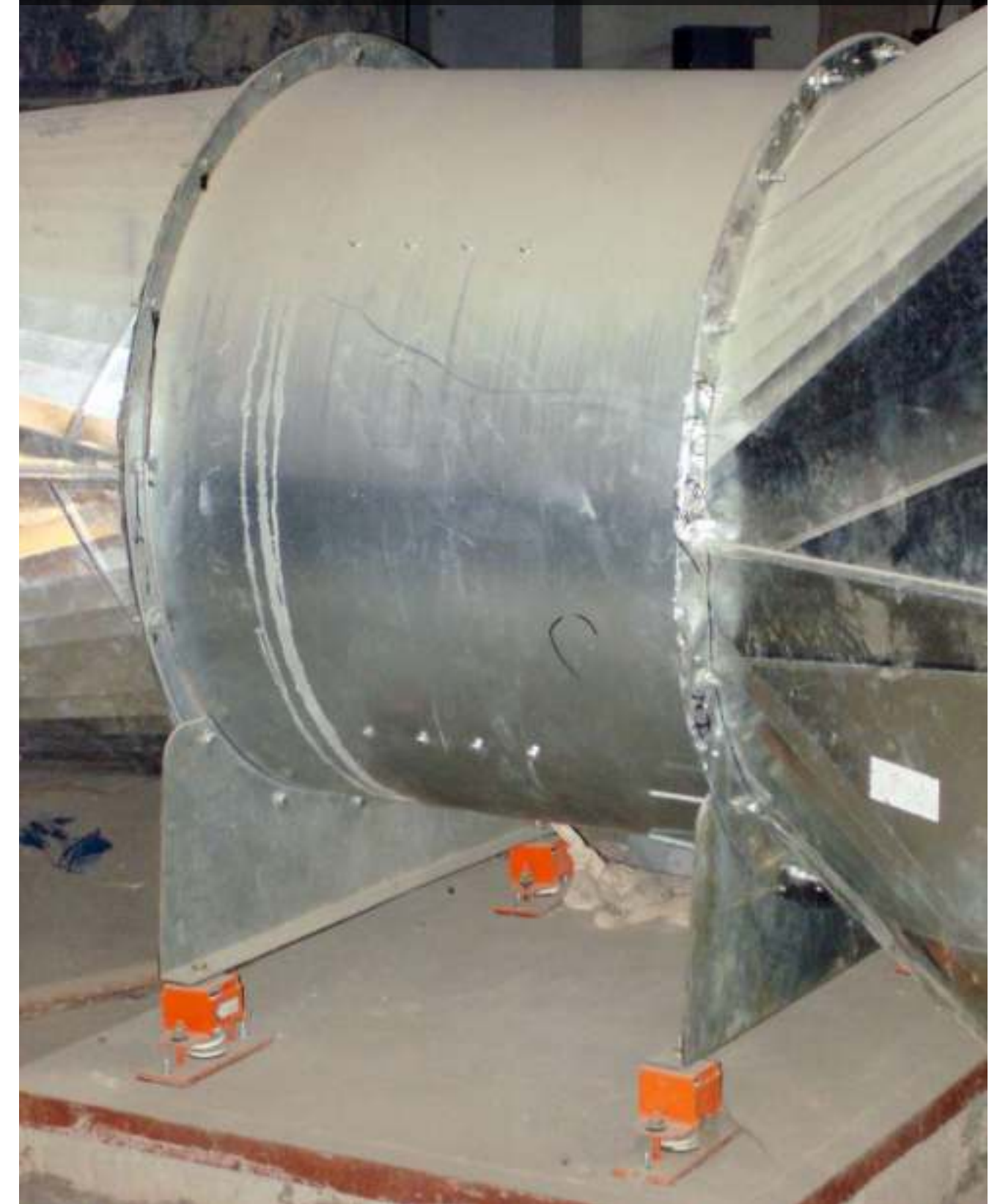
Axial Flow Fans installed with Restrained Spring Mounts
