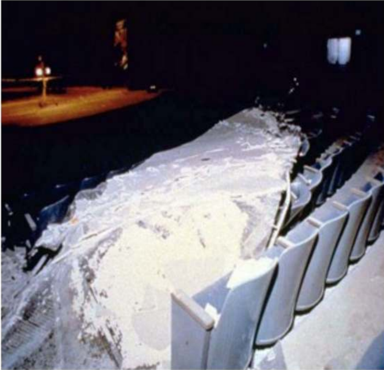
False ceiling collapsed during Earthquake
