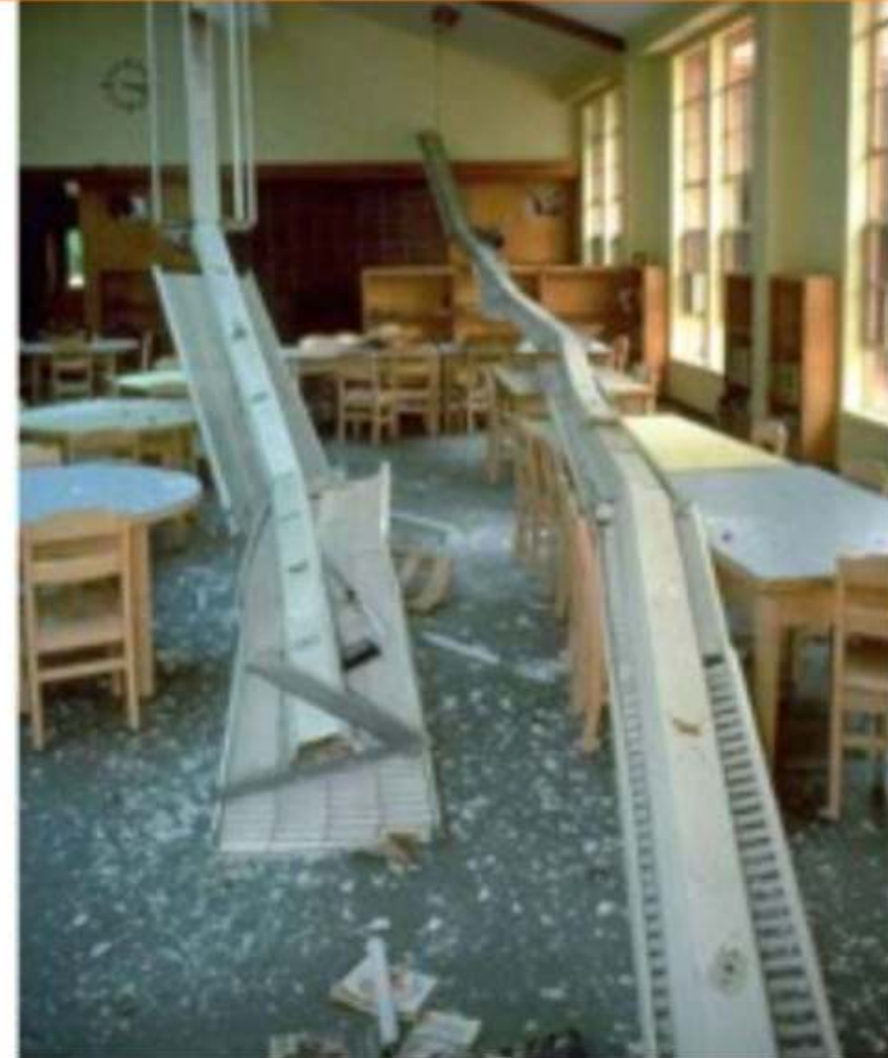
Hanging Light fixtures damaged during Earthquake
